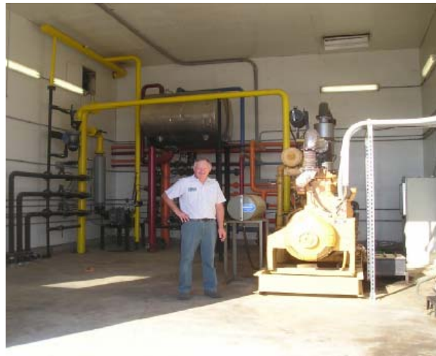
130 kW Caterpillar CHP Genset – installed 2005
