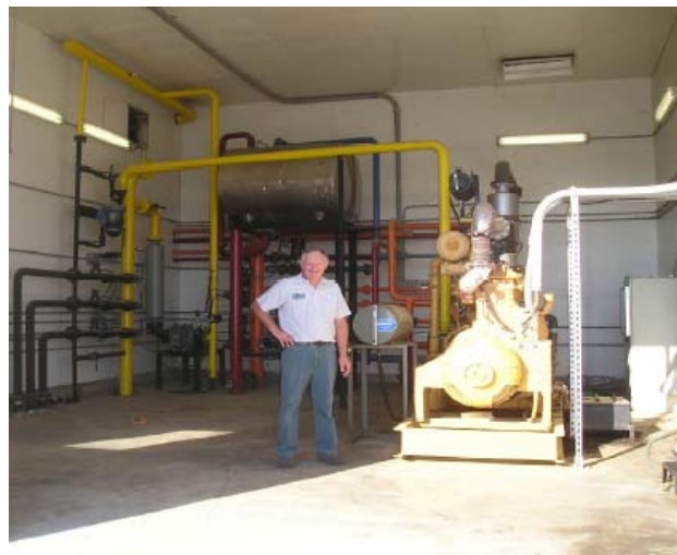
130 kW Caterpillar CHP Genset – installed 2005
