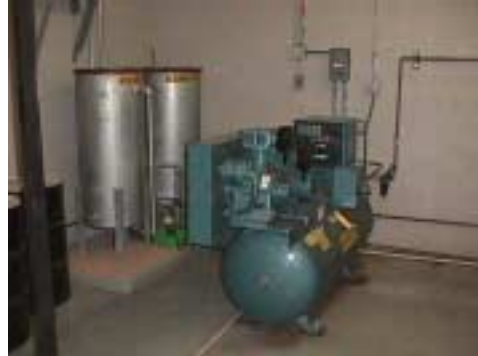
Figure 6: Blackstart® Air Compressor - Controls air compressor - Controls air compressor that runs continuously, fed by ICT emergency generator.
