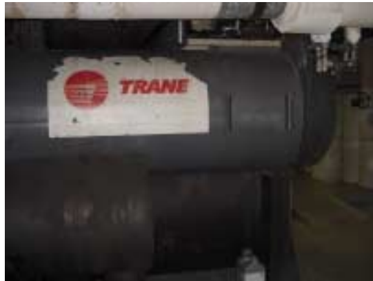
Figure 10: Trane, 550-ton, 3-stage centrifugal chiller
