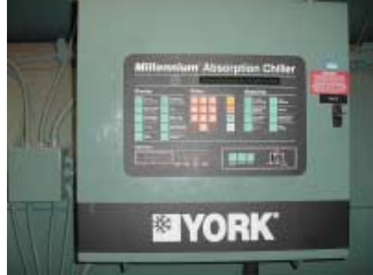
Figure 9: Controls of York Absorption Chiller
