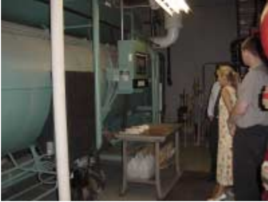
Figure 8: MAC Case study visit with Facility Operators Management Paul Dawson viewing a York 550 Millennium Absorption Chiller
