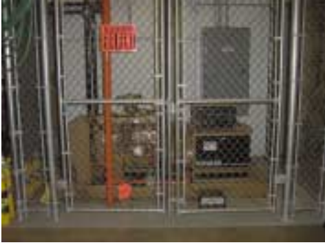
Figure 5: Kohler Emergency Generator
