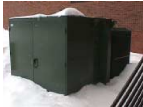
Figure 7: Winter photo of transformers rented from ComEd to step up 4,160 volts of electricity from the generators to ComEd's line of 12,470 volts.
