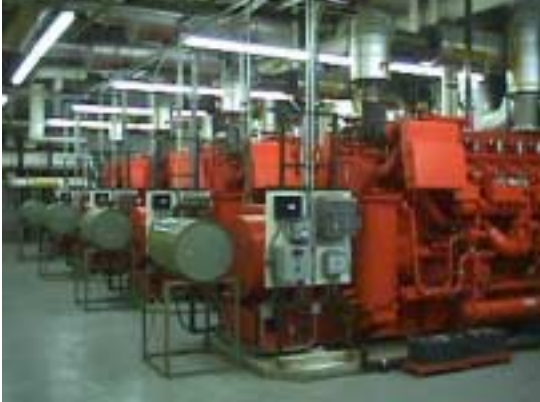
Figure 3: Waukesha engines installed at Elgin Community College
