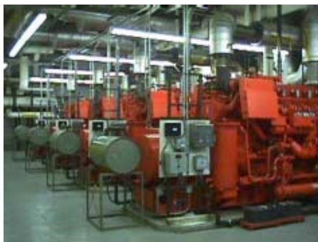
Figure 2: Four 800 kW Waukesha engines operating at ECC
