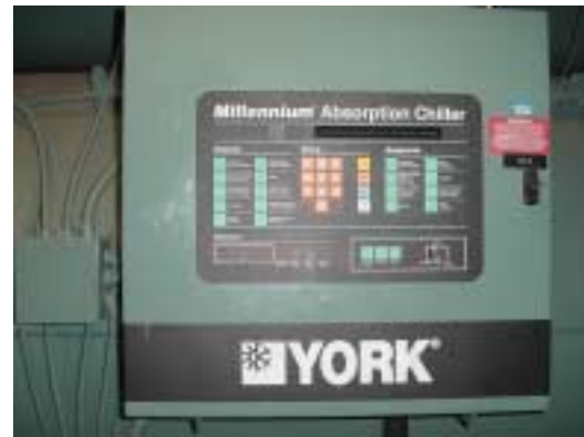
Figure 6: York Absorption Chiller Controls
